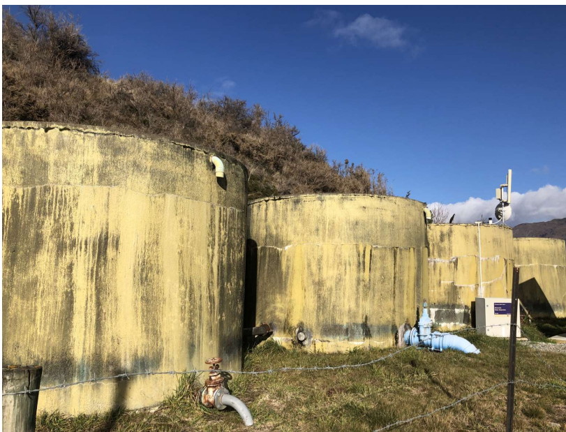
Figure 1: Existing tanks with visible cracking and water leakage
